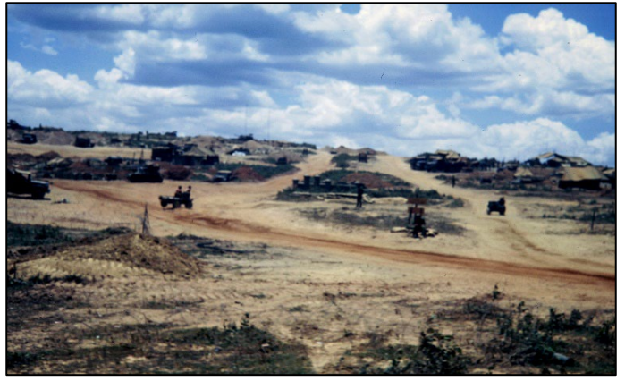
1st/44th finish building Con Thien. The most northern combat base in Vietnam. The NVA constantly attacked the base by the ground and artillery
