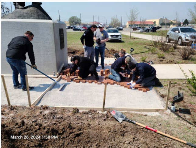
Volunteers from the ADA Warrant Officer Course help smooth the crushed rock and lay the bricks.
