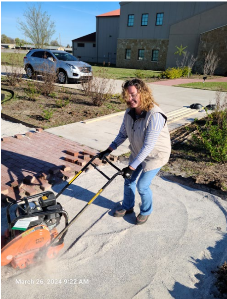
Melita Simley takes control of the soil compactor on the stone bed.
